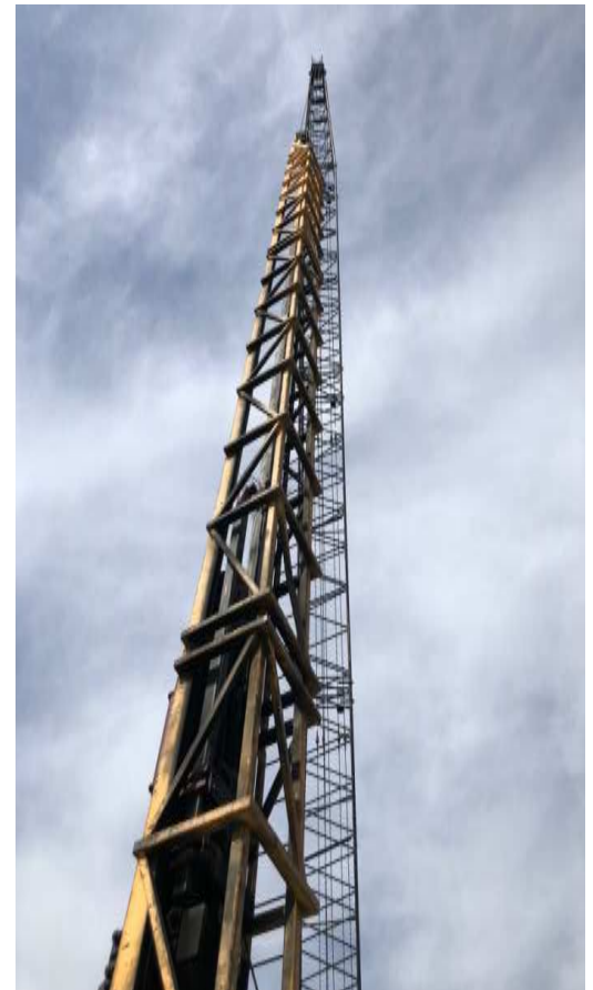
Below: Crane with the piledriver attached and ready to drive piling. Photo taken the week of April 28.
