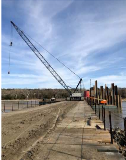
Above: Crane on the work bridge. Note the telehandler on the floating work area to the right.
